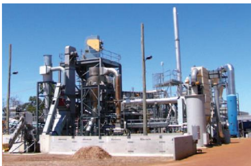
Gas-fired power plant
