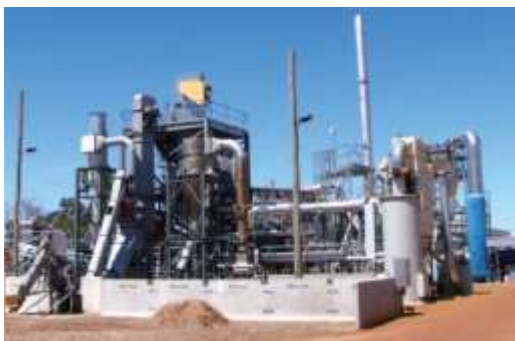
Gas-fired power plant
