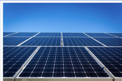
1 MW PV plant
